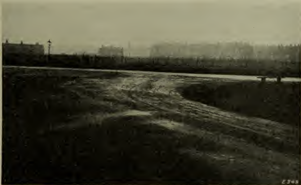
BEZA STREET, SHOWING EFFECT OF TRAFFIC ON EXPERIMENTALLY TAR-SPRAYED SURFACE.
